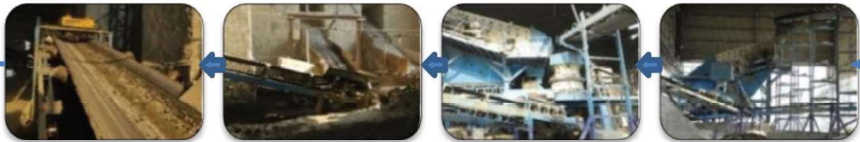
VSI Feeding Conveyor
